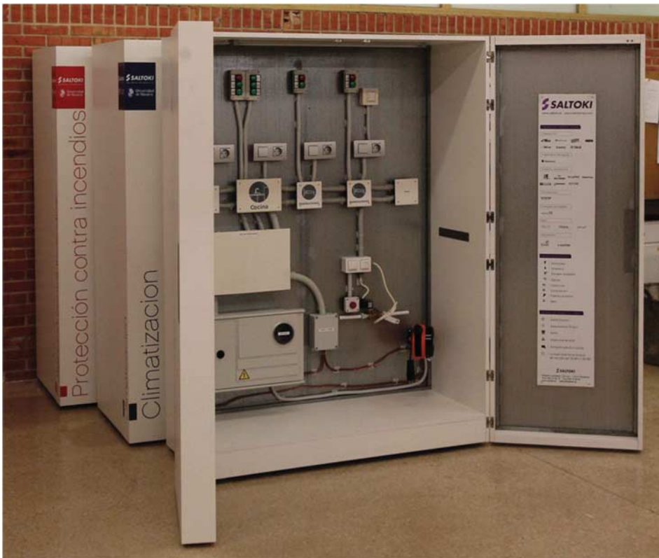
Figure 9. Technical cabinet open.
