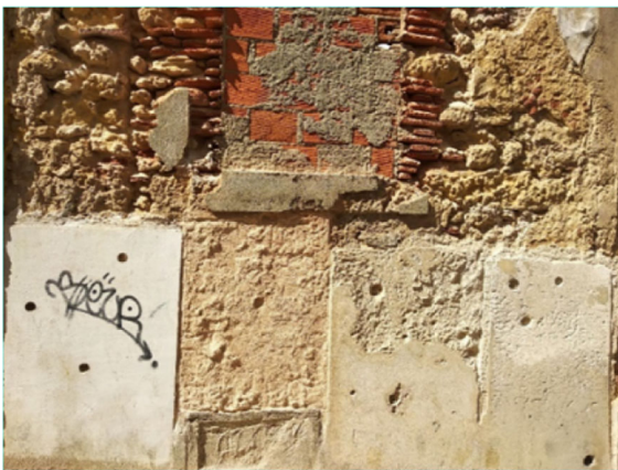
Fig. 5 Experimental panels applied on an ancient wall in the Historic Centre of Palmela (Portugal), 12 years after application: second from the left is air lime + MK and third from the left is has air lime as the only binder
