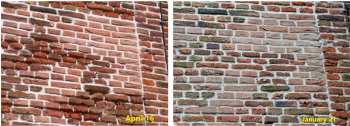
Fig. 22 Comparison of part of the south wall in April 2016 (before repair), respectively January 2021. Most of the underfired bricks are still in place (some of the weakest were replaced). The repair repointing performs rather satisfactorily
