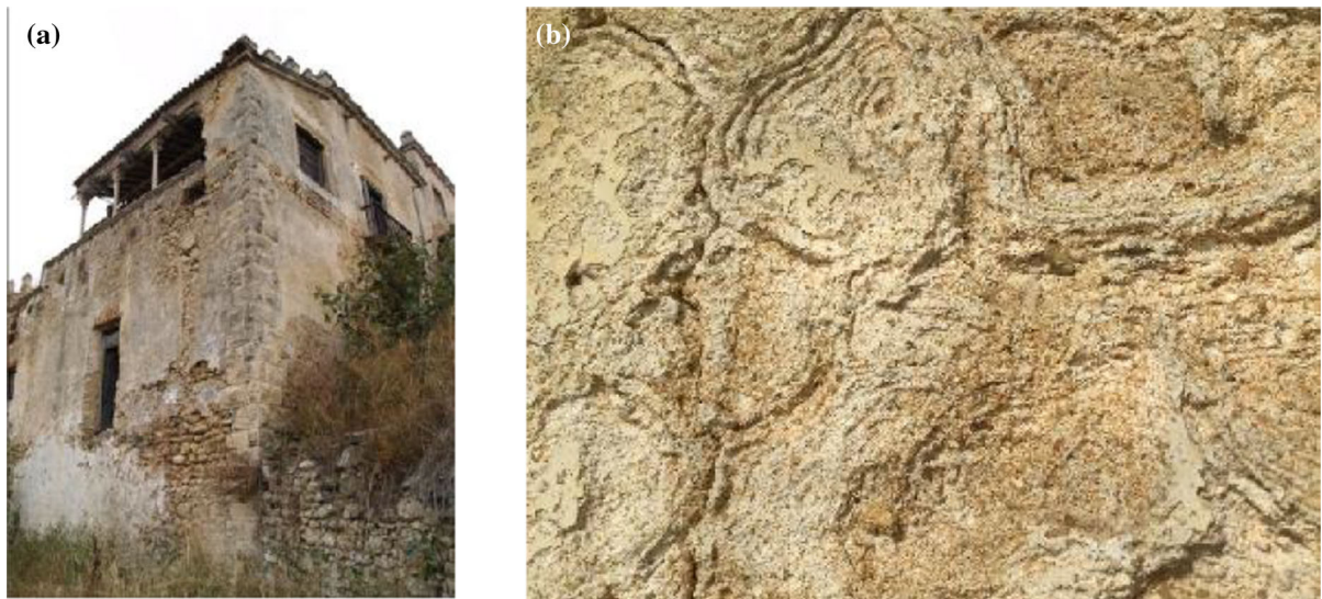
Fig. 27 Valflores Palace in St. Iria da Azoia, Loures, Portugal (a), and Liesegang phenomenon in a rendered façade (b)
