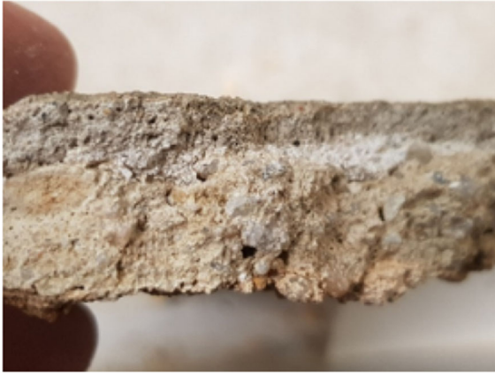
Fig. 26 Sample of the render of the East façade with a cementitious repair coat
