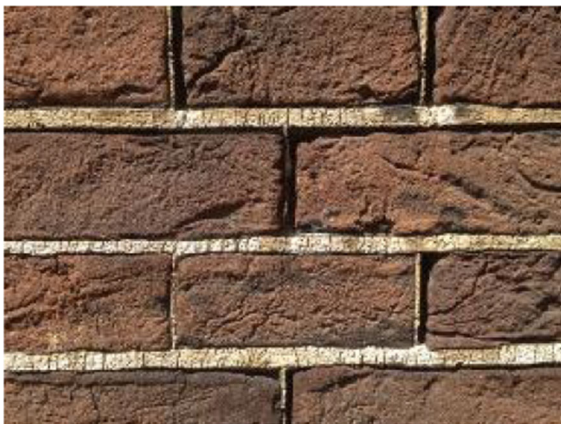
Fig. 14 Cut to shape pointing, with typically very high binder content, showing shrinkage cracks
