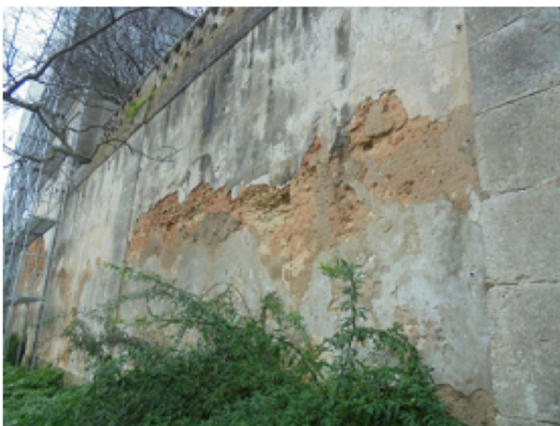
Fig. 23 Degradation on the East façade
