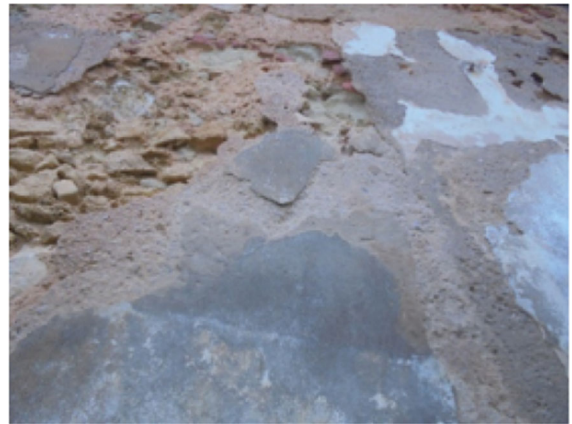
Fig. 24 Detail of the degradation showing cementitious repair mortars
