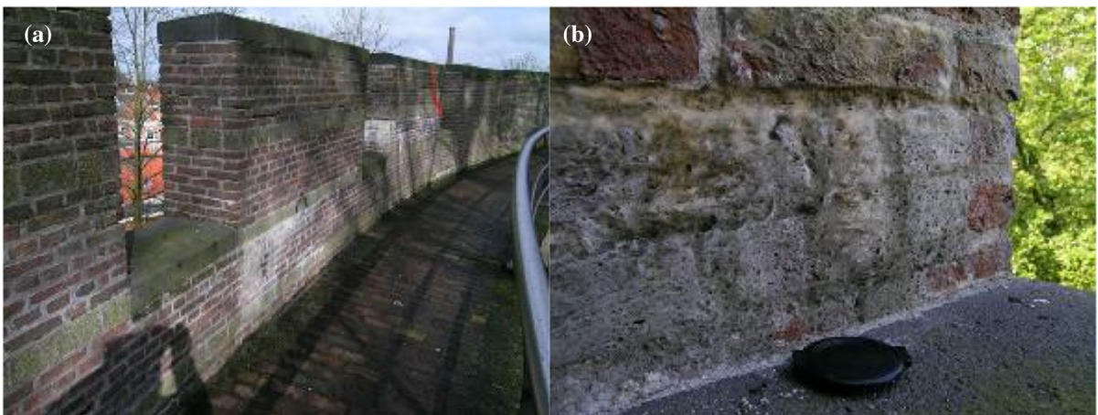
Fig. 32 a) Encrustation, due to leaching of mortar in very exposed masonry, the battlements of a motte castle; b) Detail
