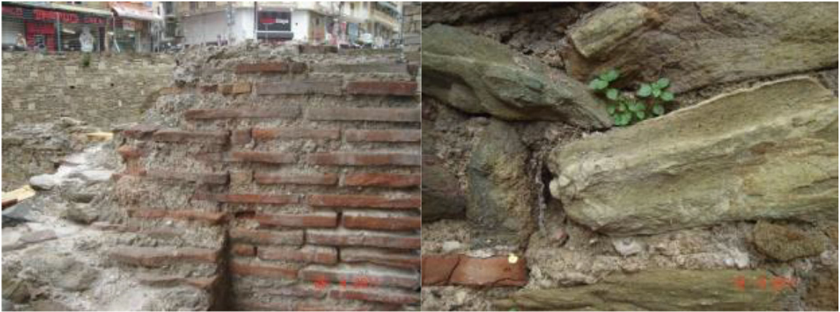
Fig. 29 Deterioration problems of the masonries before the intervention works
